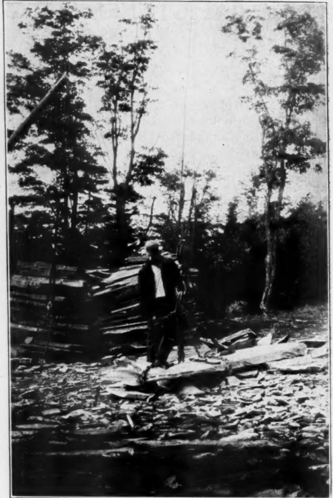
Unhooking a Block from the Steam Derrick after it has Reached to Surface
